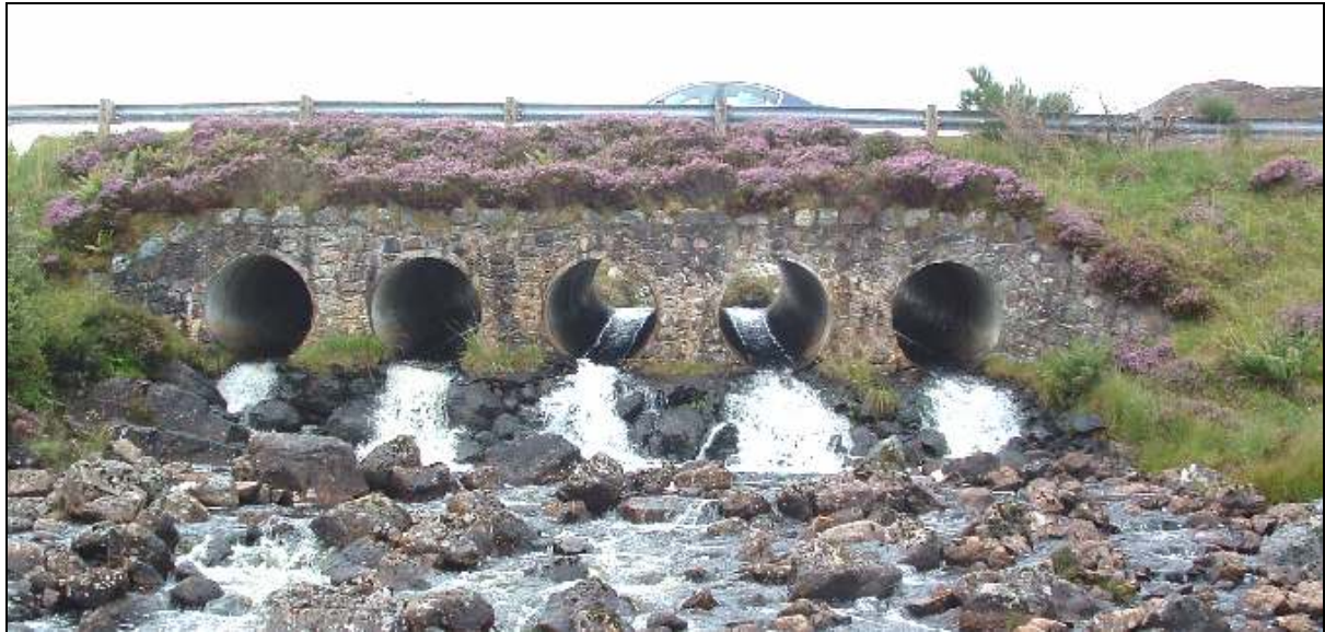
Figure 4.3.1 Impassable culvert near Second Coast
